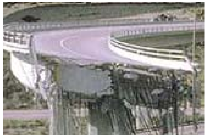
This highway in California collapsed during an earthquake. Photo Credit: USGS
